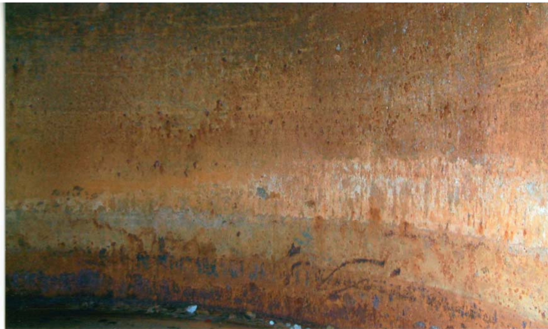
FIGURE 6 - Inside of Uncoated Holding Tank
