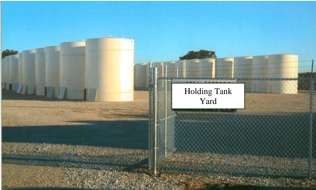
FIGURE 5 - Holding Tank Yard in Texas
