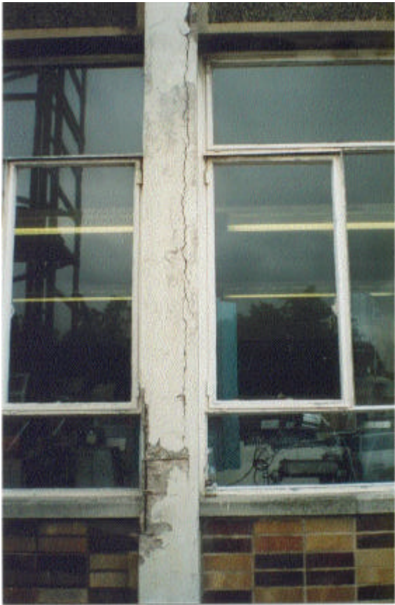
Figure 3: Typical Damage to Columns.
