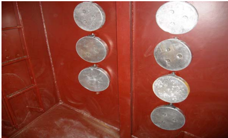
FIGURE 5 - Another View of Group F Void, 8-250-5-V with Regenerated Desiccant Containers
