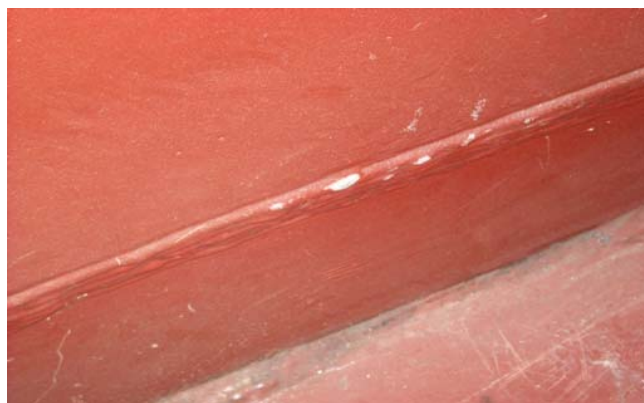
FIGURE 2 - Control Group Void, 03-143-6-V showing some areas of coating damage
