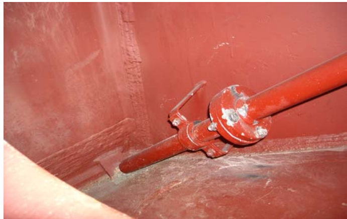
FIGURE 4 - Group F Void, 8-250-5-V showing a coating damaged pipe
