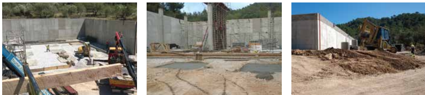
Fig 2: Progress photos taken during construction of the reservoir (photos courtesy of CAT)
