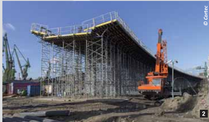
2 Bridge construction in picture above was built to have a 100 year service life. MCI®-2005 NS was used in conjunction with epoxy coated steel in the design building process to help achieve the necessary service life requirements.
