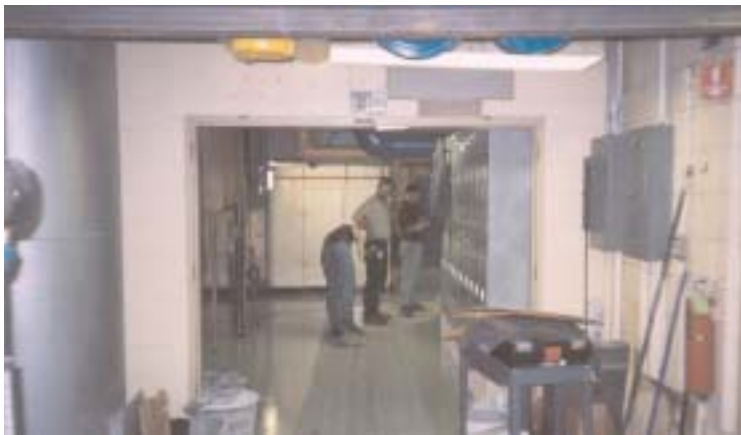
Preparation of a hospital mechanical room floor walkway for application of MCI 2026 Primer and Floor Coating
