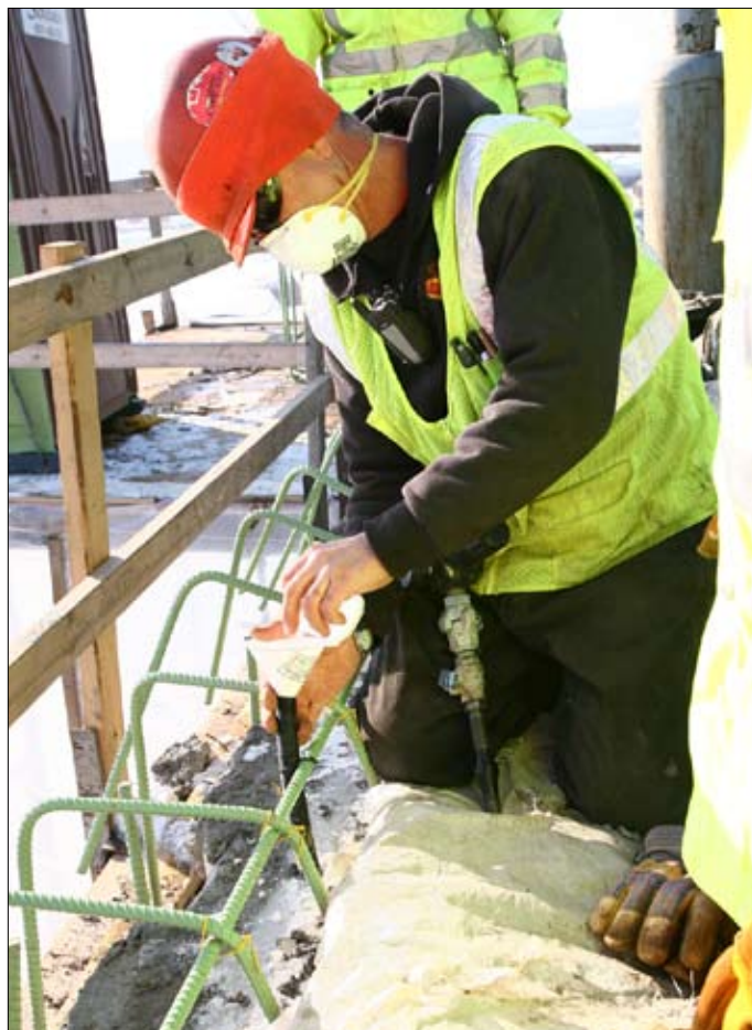
A construction worker applying MCI®-309 Powder for Post Tensioning (PT) Cables to the Wacouta Bridge in South St. Paul, Minnesota.
