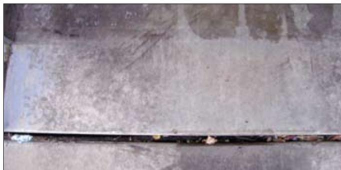
Garage floor doorway 12 hours after cleaning; MCI®-2061 was applied to the right side
