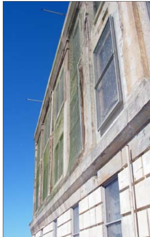
Close-up of corrosion damage
