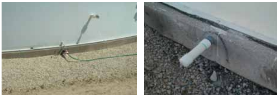
Corrosion rate monitoring probe: (a) delivering VCI slurry under the tank floor and (b) completed ER probe assembly through the ringwall.
