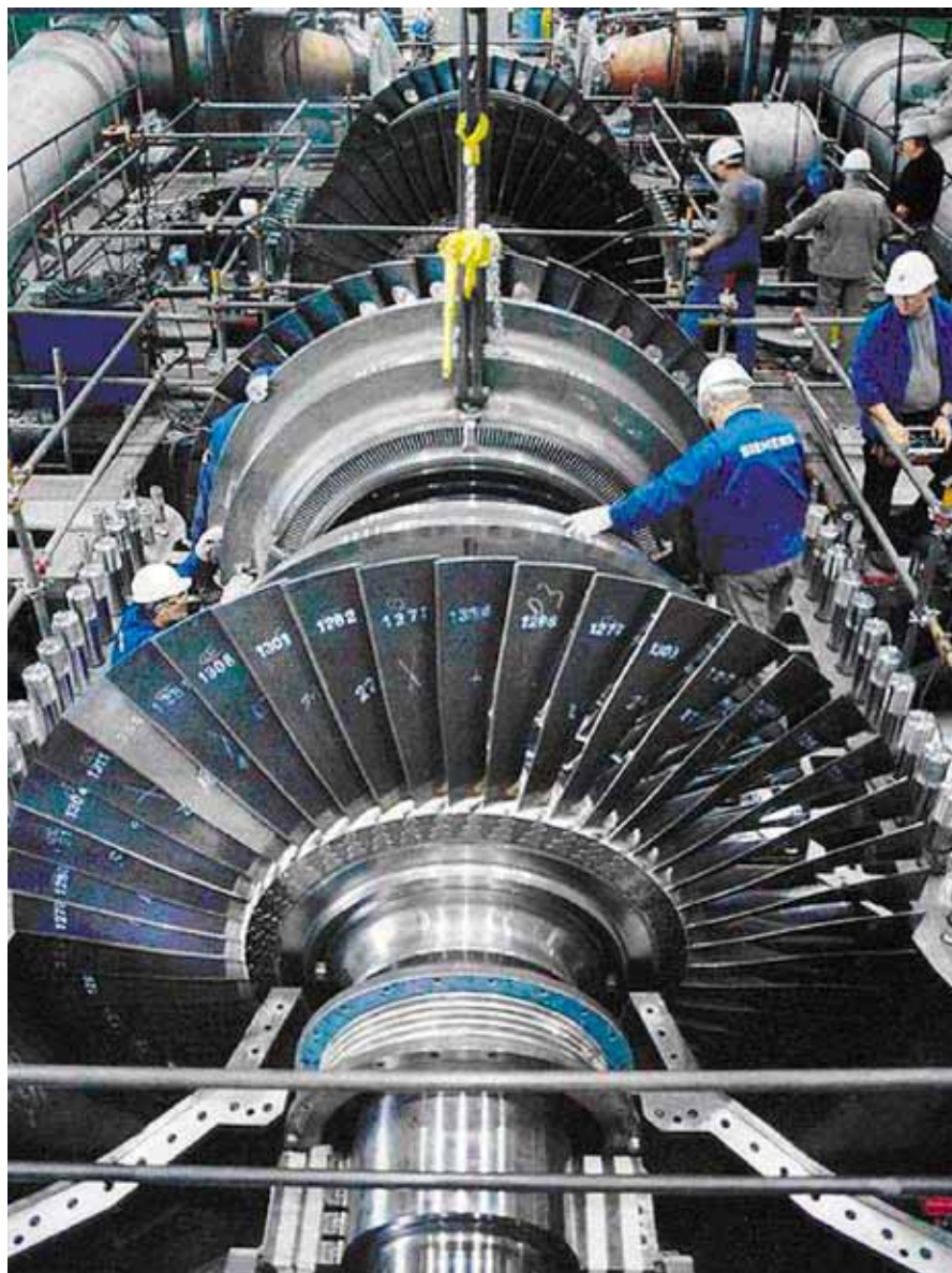
Steam turbine system.
