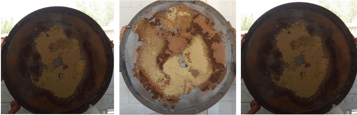
Figure 9: Underside steel plate of ICCP protected tanks at the end of pre-injection phase
