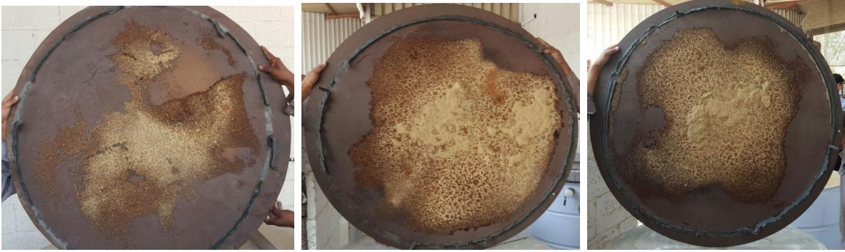
Figure 6: Underside steel plate of unprotected tanks at the end of pre-injection phase
