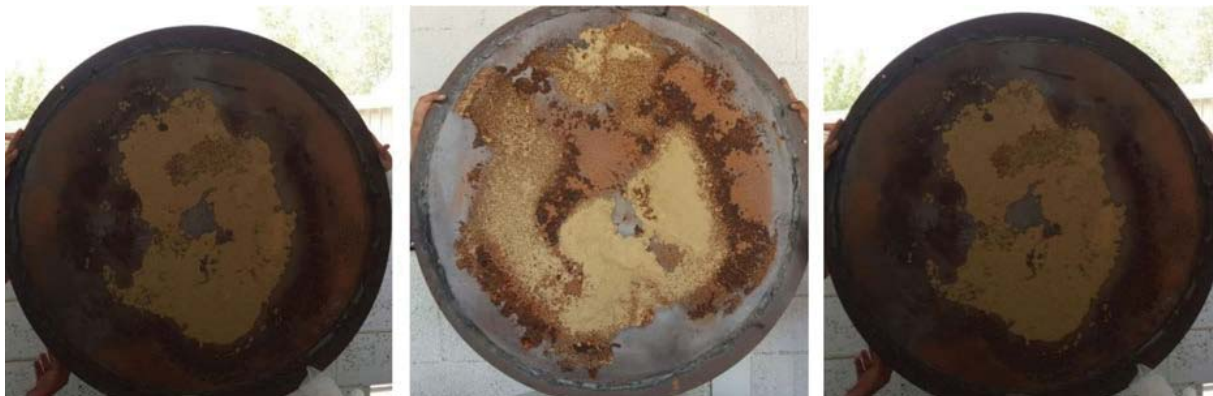
FIGURE 9. Underside steel plate of ICCP-protected tanks at the end of pre-injection phase.
