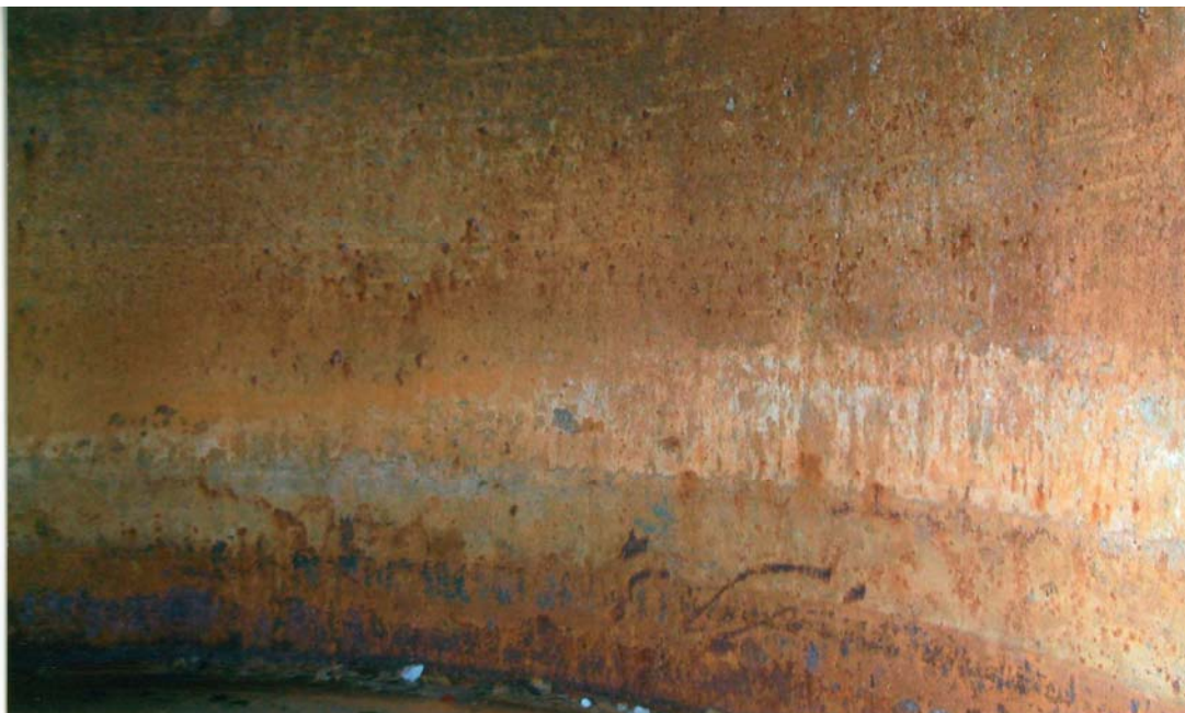
FIGURE 6 - Inside of Uncoated Holding Tank
