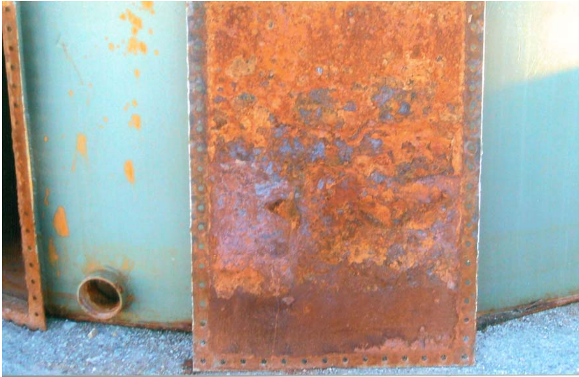
FIGURE 7 – Uncoated Holding Tank Hatch
