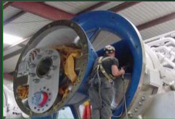
Fogging through the inlet
