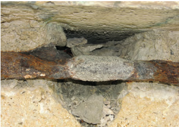
Zagreb Cathedral – damaged steel joints on south tower.
