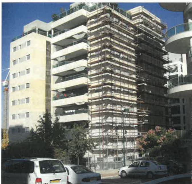
Fig. 1: Stav Street residential building during repairs (image courtesy of Glimmer Industrial Consultation)
