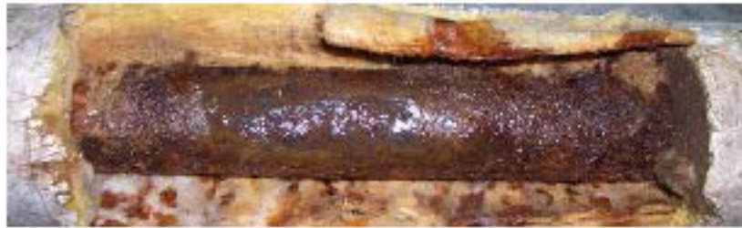
An example of the deteriorated condition of an existing pipe with CUI.
