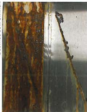
FIGURE 2—Corrosion on traditional water-based coating (left) vs. minimal creepage corrosion from scribe on panel coated with 1 mil of NANO-VCI water-based coating (right) after 1,000 hours of salt spray exposure.
