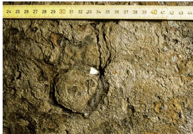
Figure 1. Microbiologically induced corrosion of product storage tank bottom plate after 6 years (CASE HISTORY 01.11.17.01) [8]
