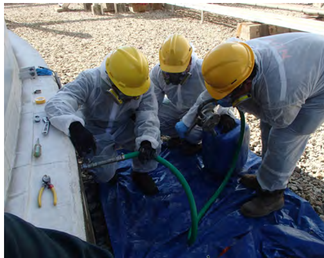
Figure 4. Injection of CorroLogic Slurry beneath an in-service storage tank. Image courtesy of Cortec Southeast Asia.
