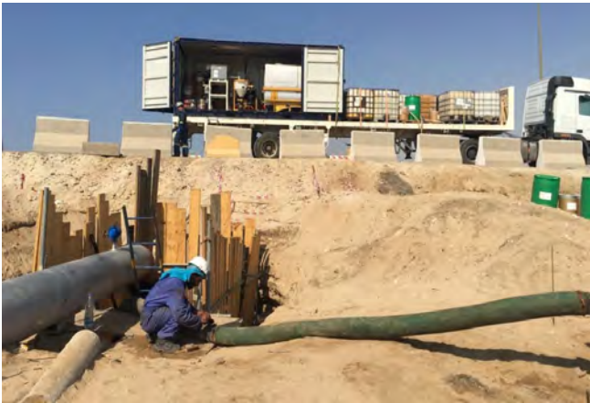
Figure 1. Aboveground pipelines are redirected underground at road crossings and placed in casings to protect them from the weight of the road. CP is generally not viable here; however, CorroLogic® VpCI® Filler presents an exciting alternative protection option. Image courtesy of Cortec® Case History 628.
