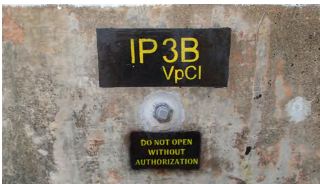
Figure 3. Holes were drilled (and later sealed) to allow injection of VpCI in the form of CorroLogic Slurry. Image courtesy of Cortec Southeast Asia.
