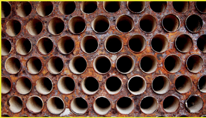
Pixabay (credit Nickbar) image for illustration only as an example of what happens when hydrotesting is not done properly.
