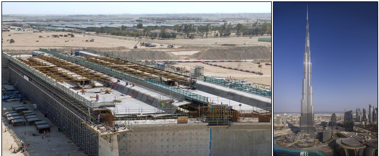
Image 1. MCI® powder was injected into post tensioned ducts just after placement of post tension cables. This decreased time and expense needed for corrosion protection of the orbital high way. Image 2. Especially significant example of using MCI® and design life modeling to extend service life is the Burj Khalifa tower.
