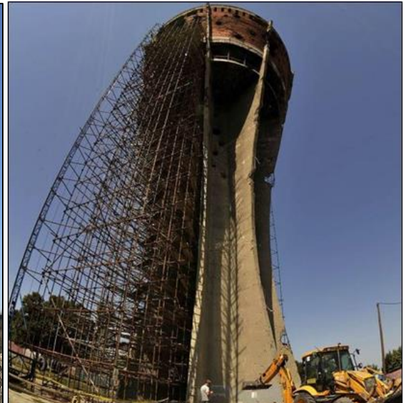
CorrVerter MCI® was applied recently during preservation of Croatian, war-destructed water tower monument.
