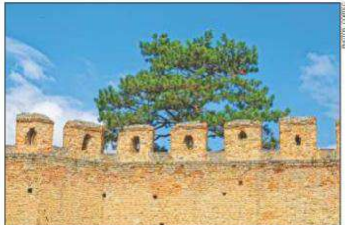
The walls are exposed to damaging atmospheric influences, and the binding material between the bricks has washed away, leading to brick deterioration.
