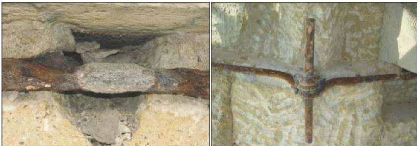
The joints were reinforced with steel fishplates that were welded onto the joints and also protected with CorVerter® MCI® Rust Primer.
