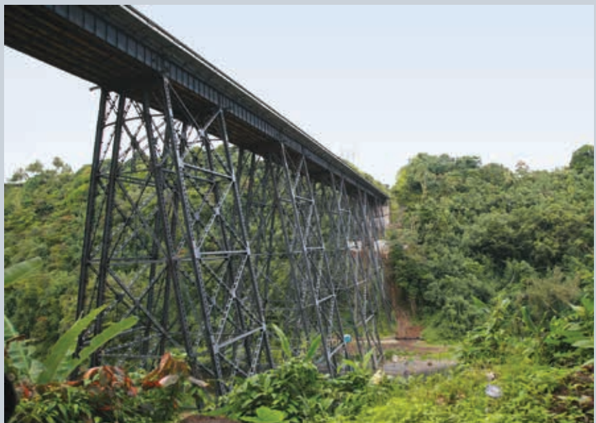
Workers can clean away loose rust, apply CorrVerter® to passivate and protect the surface, and use VpCI®-384 as a heavy-duty topcoat.
