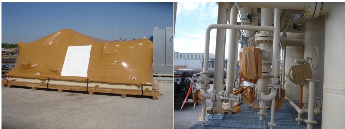
The equipment, pipes, flanges, and units wrapped in MilCorr® VpCI® Shrink Film. A heat gun was used to complete the shrink-wrapping process during preservation.
