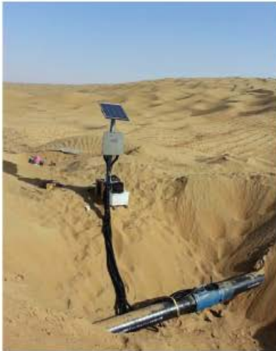
↑ Non-intrusive Field Signature Method corrosion monitoring of a pipeline powered by solar panels.
