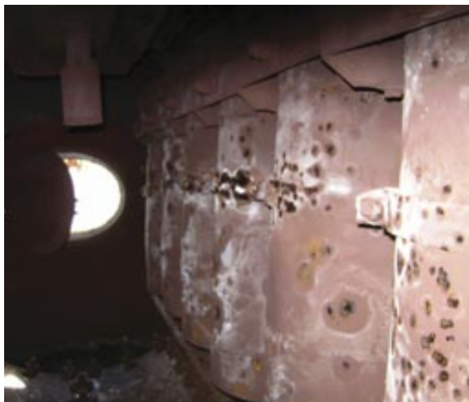
Pitting corrosion on steam drum separators, likely caused by a deficient wet layup. Cortec® image.
