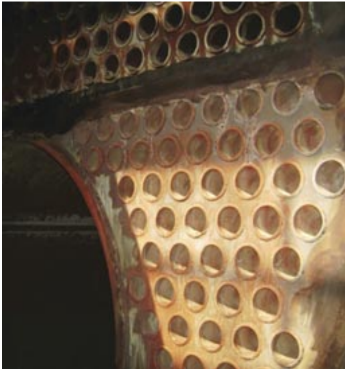
Orange/reddish color in the tube sheet of a firetube boiler suggests some corrosion has occurred in the fireside. Cortec® image.
