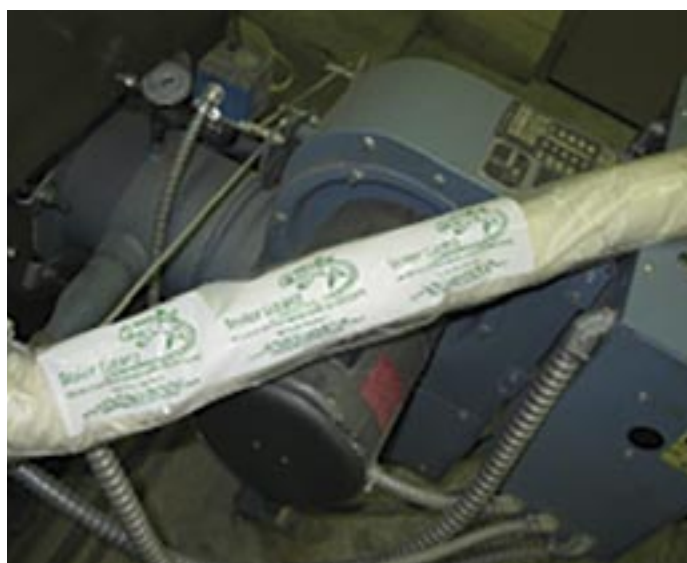
A classic example of VCI dry layup: VCI powders packaged in a water-soluble tube that dissolves when the boiler is refilled. Cortec® image.
