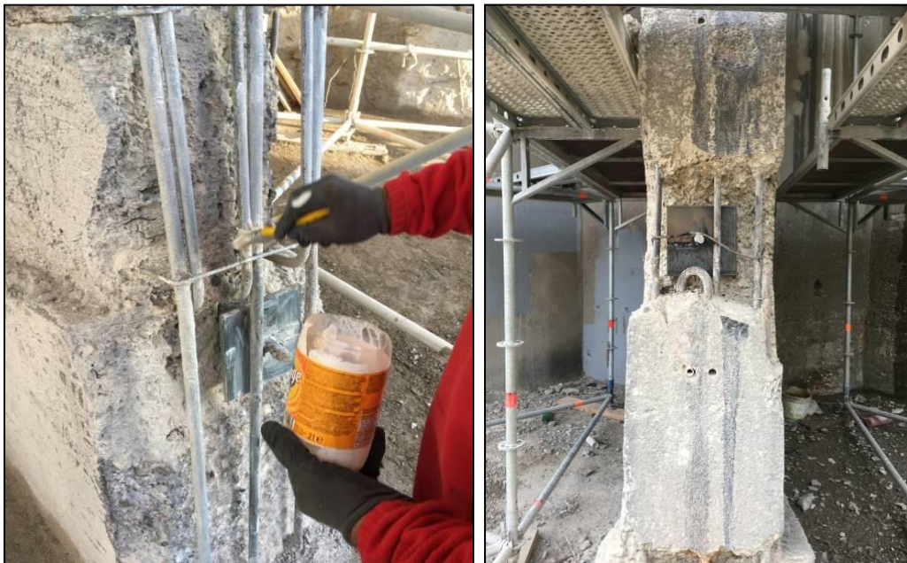
CorrVerter® MCI® was applied to heavily corroded metal surfaces of the water tower. They have been unprotected and rusting for over 20 years since the war ended.
