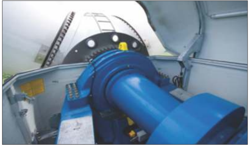
Modern wind turbines may comprise 1000 or more bolts that undergo rigid maintenance system.
