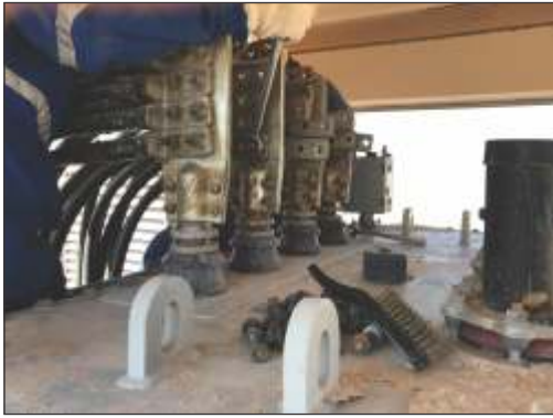
Corroded clamps in the transformer box were washed with VpCI®-415 and dried. ElectriCorr® VpCI®-239 was applied and they were bolted back into place. VpCI®-386 was used on the clamp external surfaces.
