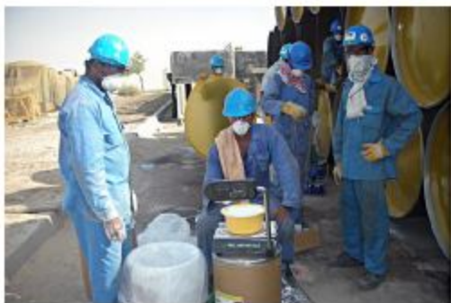
Figure 3. Pipes were sealed with an end cap and Cortec VpCI-309 powder was fogged in at a rate of 500 g/m 2 .
