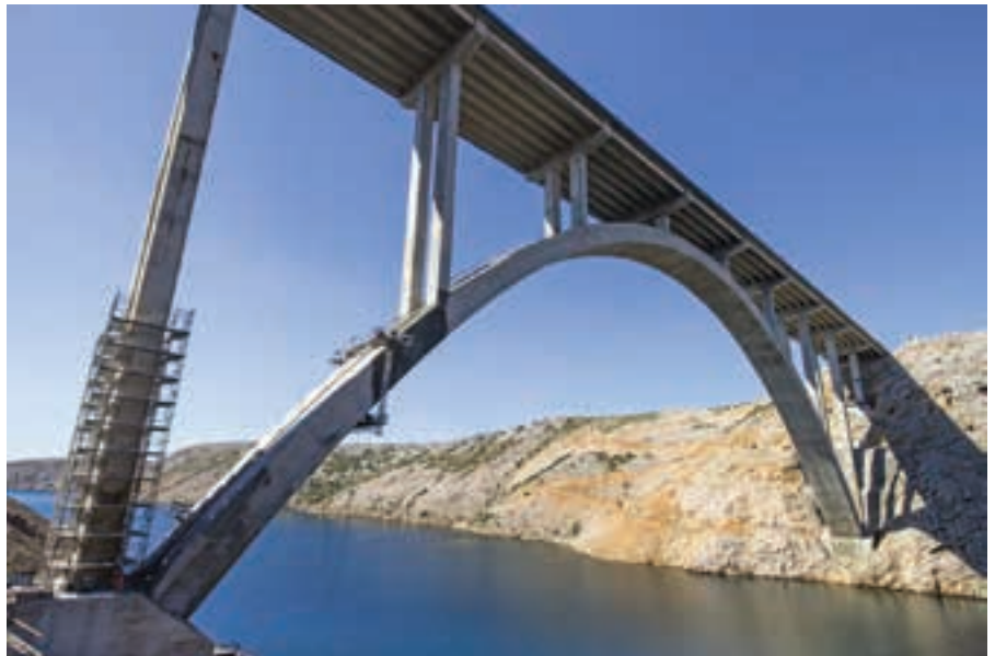
The Krk Bridge in Croatia, where Cortec's MCI 2020 surface applied corrosion inhibitor was selected to treat salt damage.
