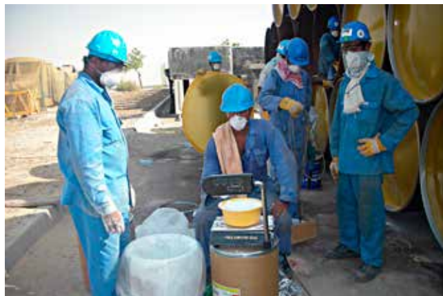
Figure 3. Pipes were sealed with an end cap and Cortec VpCI-309 powder was fogged in at a rate of 500 g/m 3 .
