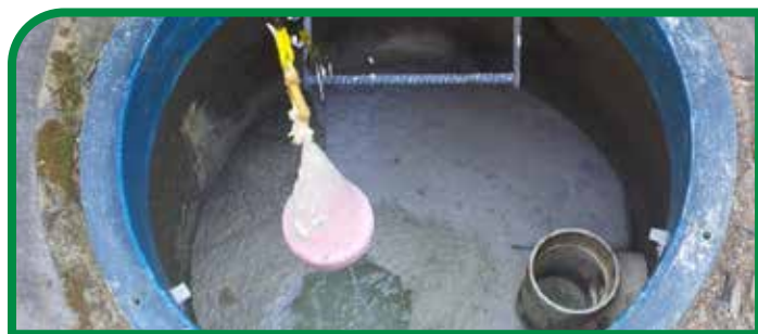
SOLVING GREASE TRAP PROBLEMS AT CHEESE FACTORY Bionetix® Case History #49
