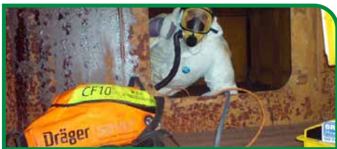
BOILER LAYUP DURING POWER PLANT MAINTENANCE OUTAGE Case History #649
