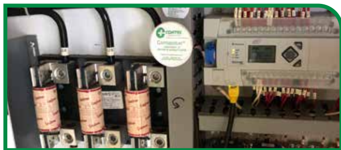
PROTECTING ELECTRONICS PANELS IN WASTEWATER PUMPHOUSES Case History #669
