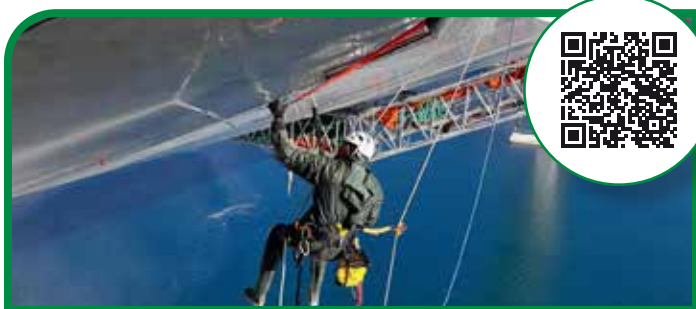
PELJESAC BRIDGE PROTECTION Case History #746
