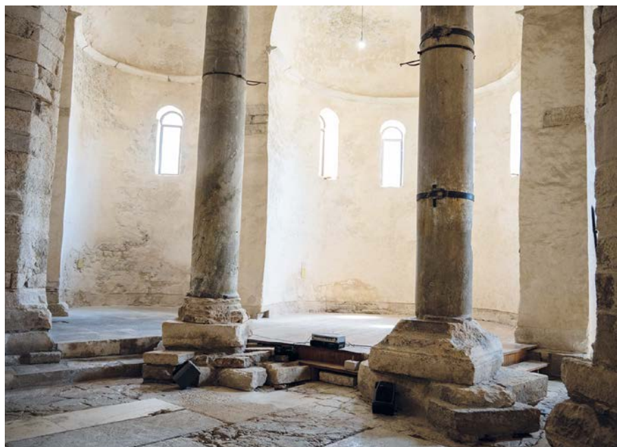
Moisture penetrating into the medieval monument, combined with airborne sea salt, poses a serious threat to the reinforced concrete structure that supports the Church of St. Donatus
