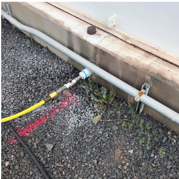
Figure 1. Single bottom tank at US East Coast tank farm received VCI injection through ports drilled in the concrete ring wall (image courtesy of Shane Baker).
