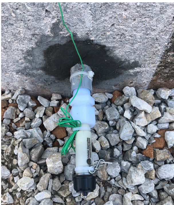
Figure 2. ER probe placed after VCI injection to continue monitoring corrosion potential readings under the tank (image courtesy of Shane Baker).
