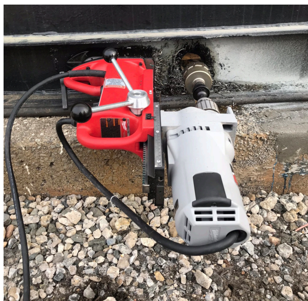
Figure 3. Drilling VCI injection ports for double-bottom tank. Two parallel horizontal lines show the locations of the original floor (lower line) and the newest floor (top line) (image courtesy of Shane Baker).
