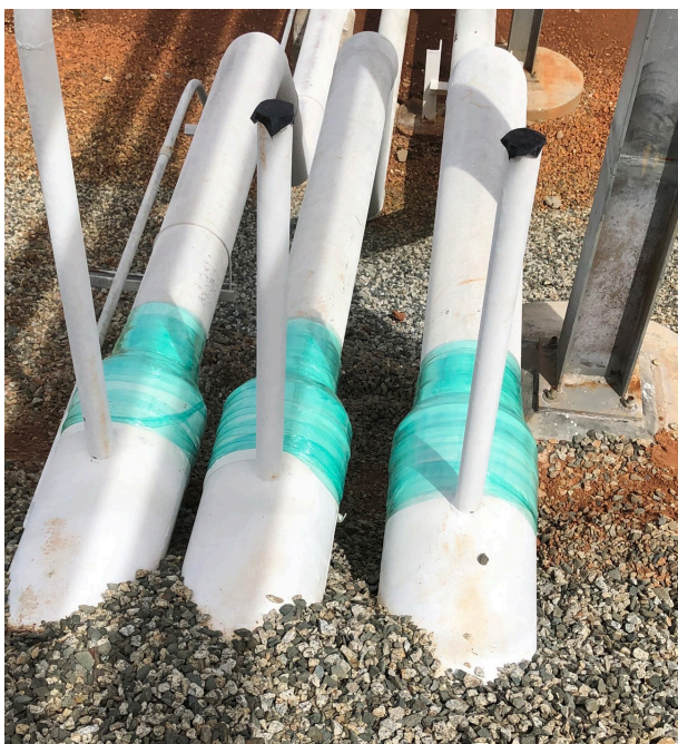
Figure 5. VCI was also injected into casings where tank farm pipelines were buried underground (image courtesy of Shane Baker).
